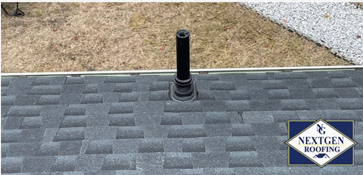
Nextgen Roofing installations of The Ultimate Pipe Flashing® and The Ultimate Bath/Dryer vent.
