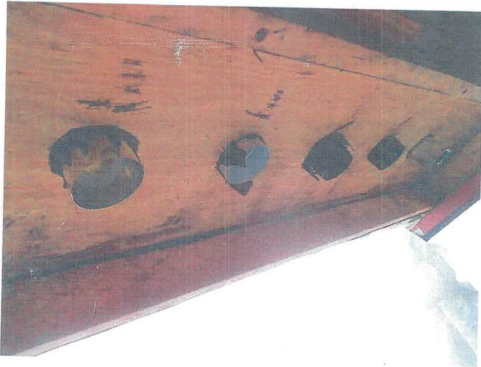
BELOW DECKING WITH 4" DIAMETER EXTENDED PIPING
